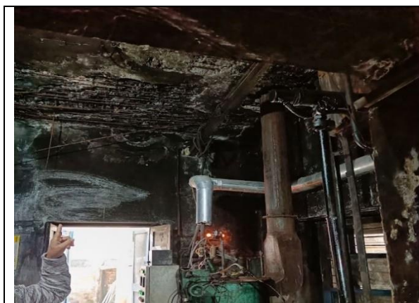
Deteriorated roof in building at Nagrotta
